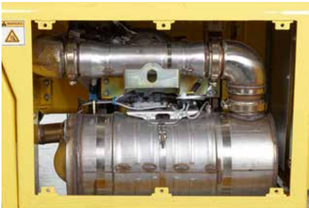
After treatment access with vent (top) and without vent (bottom)
