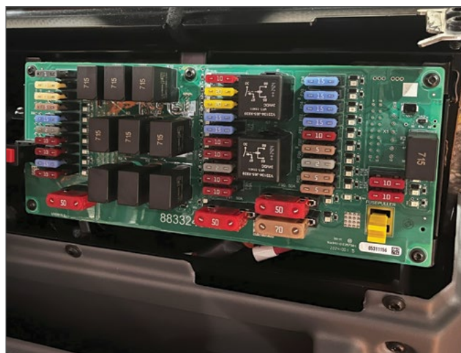
Fuse warning lights
